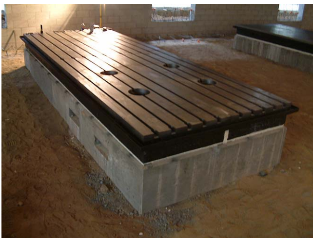
View on base plate on seismic mass showing the access tunnels through the seismic mass and base plates.
